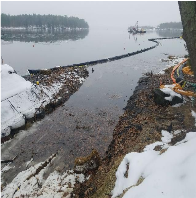
Fig 19: Turbidity barrier at Gundalow landing/east side of the Bay. Viewing west. (12-09-19).
