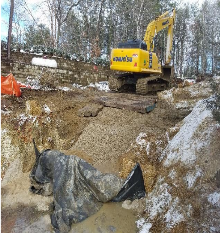
Fig 29: Crushed stone added to Gundalow landing/east side of the Bay. Viewing east. (12-11-19).
