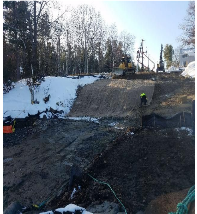
Fig 14: Restoration of slope at Getchell property/west side of the Bay. Viewing west. (12-07-19).
