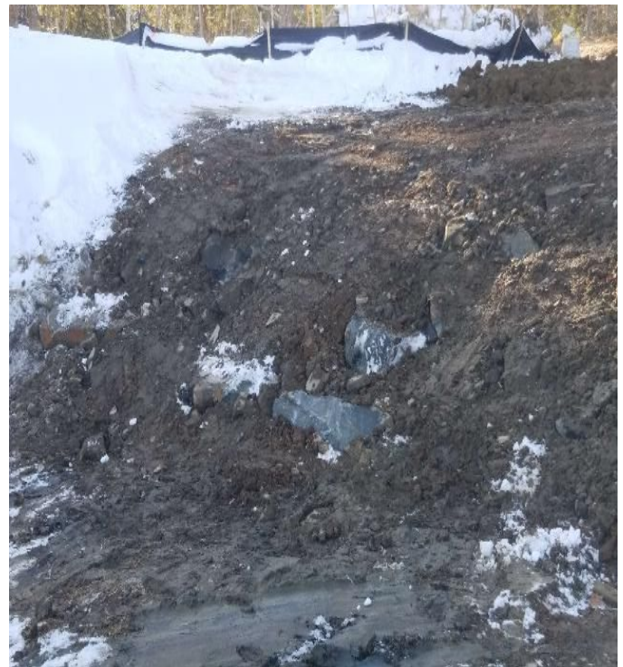
Fig 12: Large diameter boulders placed to stabilize toe of slope at Getchell property/west side of bay.. Viewing west. (12-07-19).
