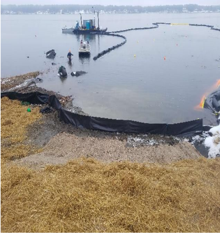
Fig 21: Restored slope at Getchell property/west side of the Bay, making adjustments to turbidity barrier. Viewing east. (12-09-19).
