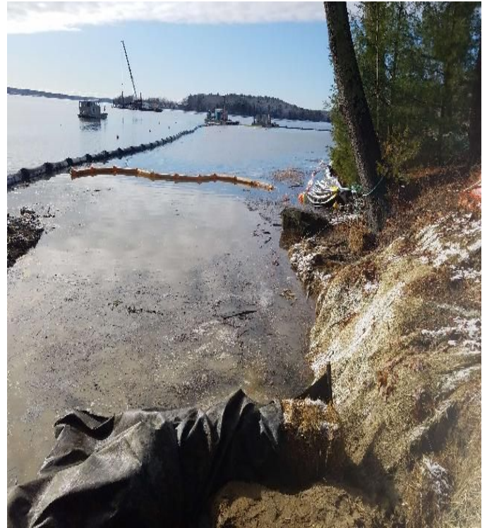
Fig 30: Crews installing silt curtain at Gundalow landing/east side of the Bay to contain sediment discharge. Viewing west. (12-11-19).
