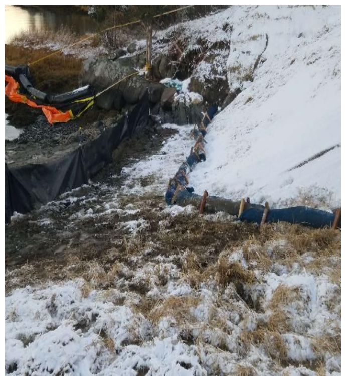
Fig 32: Filter sock installed at toe of slope at Getchell property/west side of the Bay. Viewing south. (12-11-19).
