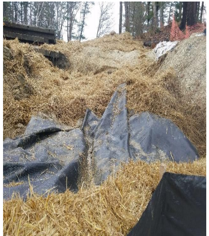
Fig 26: Crew re-installed sediment controls at Gundalow landing/east Side of the Bay. Viewing east. (12-10-19).
