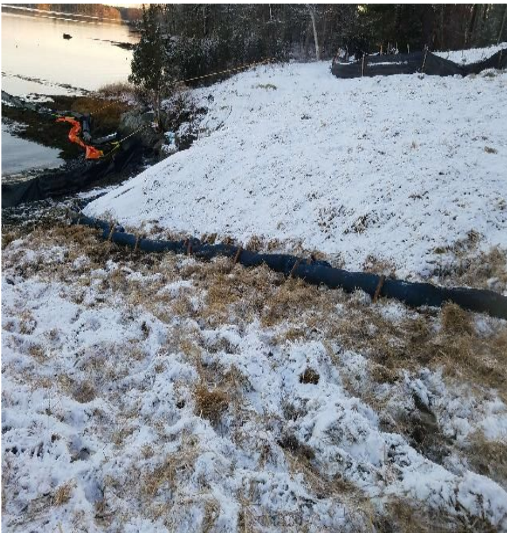
Fig 31: Filter sock installed at toe of slope at Getchell property/west side of the Bay. Viewing south. (12-11-19).
